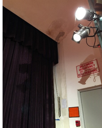
Auditorium upgrades will include repairs of interior areas damaged due to leaks prior to roof replacement.
