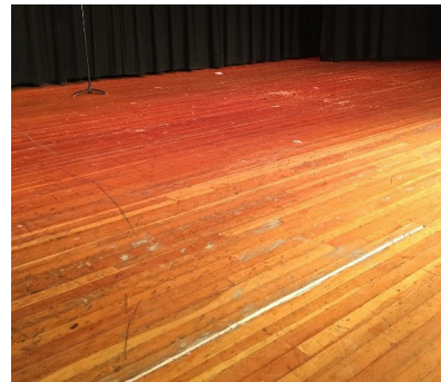
The current auditorium wood stage is too thin to refinish. The current cracks have been patched for several years in order to keep the surface safe. The current stage curtains will need to be removed in 2019 when the current fire retardant certificate expires. They are not able to be re-treated due to their poor condition.
