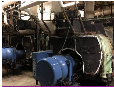
The Main Street campus is heated by two steam boilers installed when the building was built in 1958. The boiler shells have had multiple crack repairs over the last few years.
